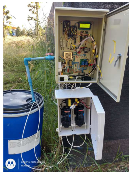
Fig. 8. control cabinet and fog pump cabinet
